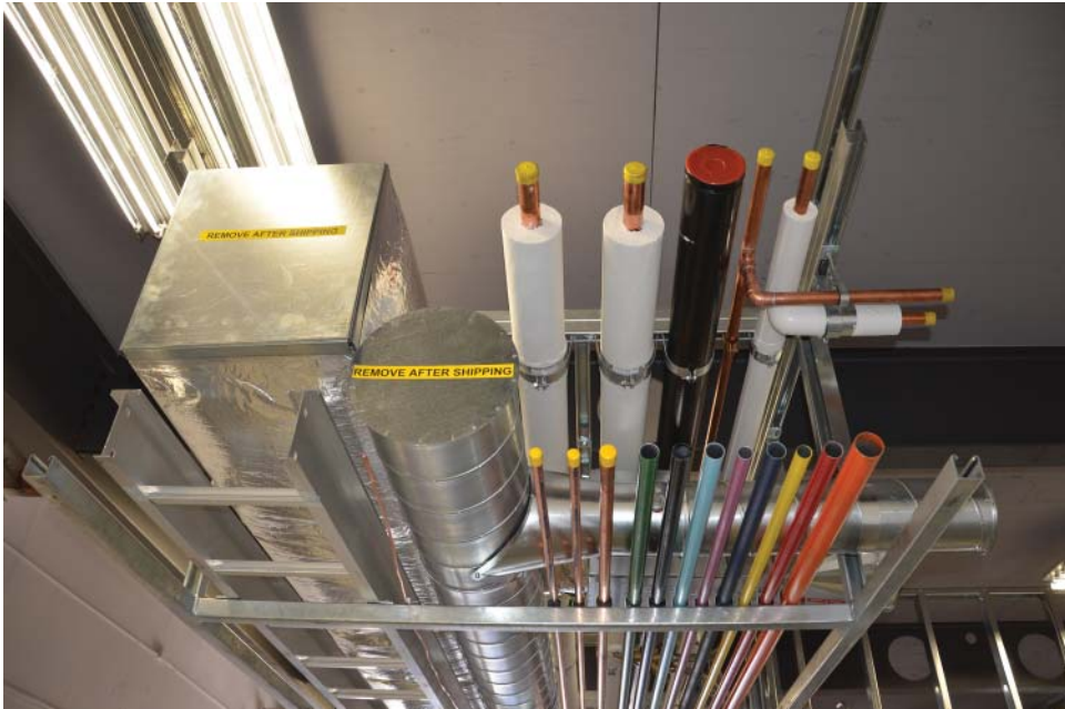
FIGURE 7.18 Installed rack similar to the prototype sections. © Southland Industries.
