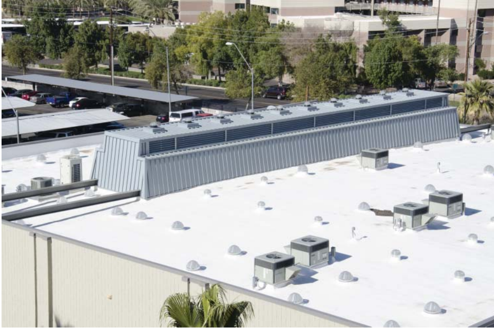
FIGURE 4.5 The solar chimney. Gregg Mastorakos; courtesy DPR Construction and SmithGroupJJR.
